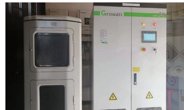
A power storage system that reuses End-of-life HEV batteries
